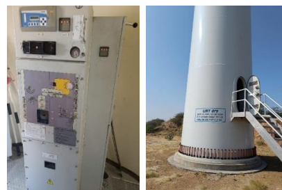
36kV GIS Installation - Wind Farm
